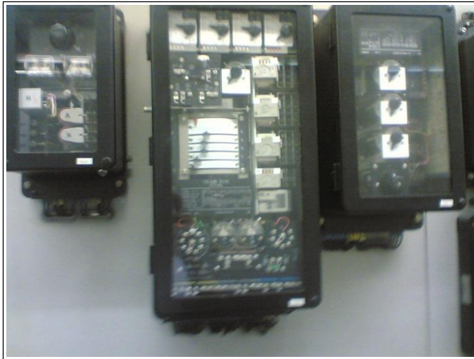
Fig. 2. Electromechanical relay for a feeder.
